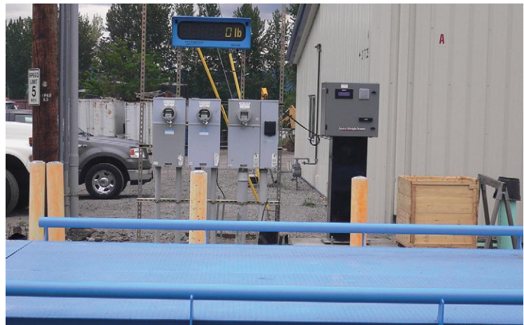
At Peninsula Terminal's transfer site, a scale system featuring high capacity, rugged construction and guardrails for additional safety provides high-accuracy weighing in a challenging climate.
